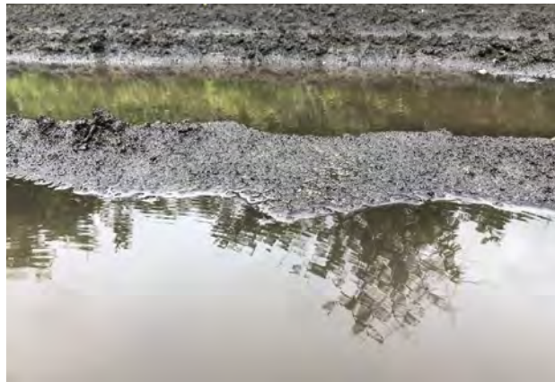
Figure 14: Poor Drainage: low area with clay soil
